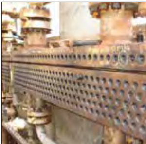
FinFan cooler before maintenance
