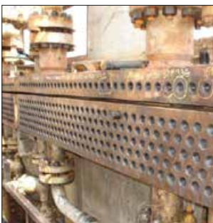
FinFan cooler before a maintenance
